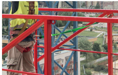
Safety points for attaching personal protective equipment.
